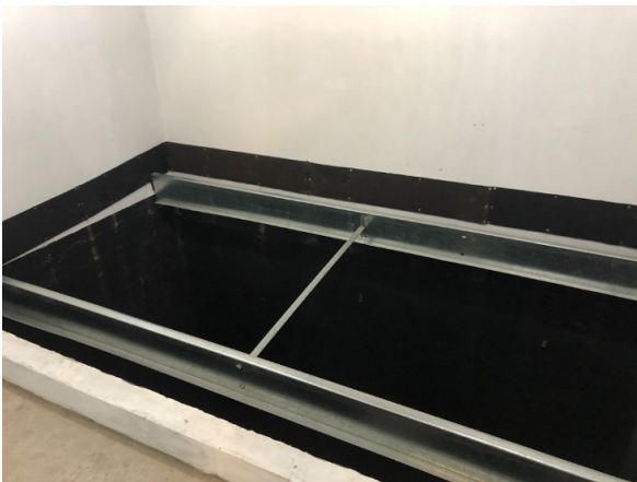
Figure 2: Space for sample installation.
